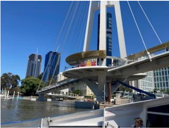
Brisbane's newest foot bridge from The Gardens to Kangaroo Point nears completion.
